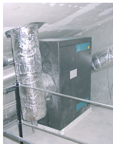
Figure 11 Insulation of ductwork, source: PHI
